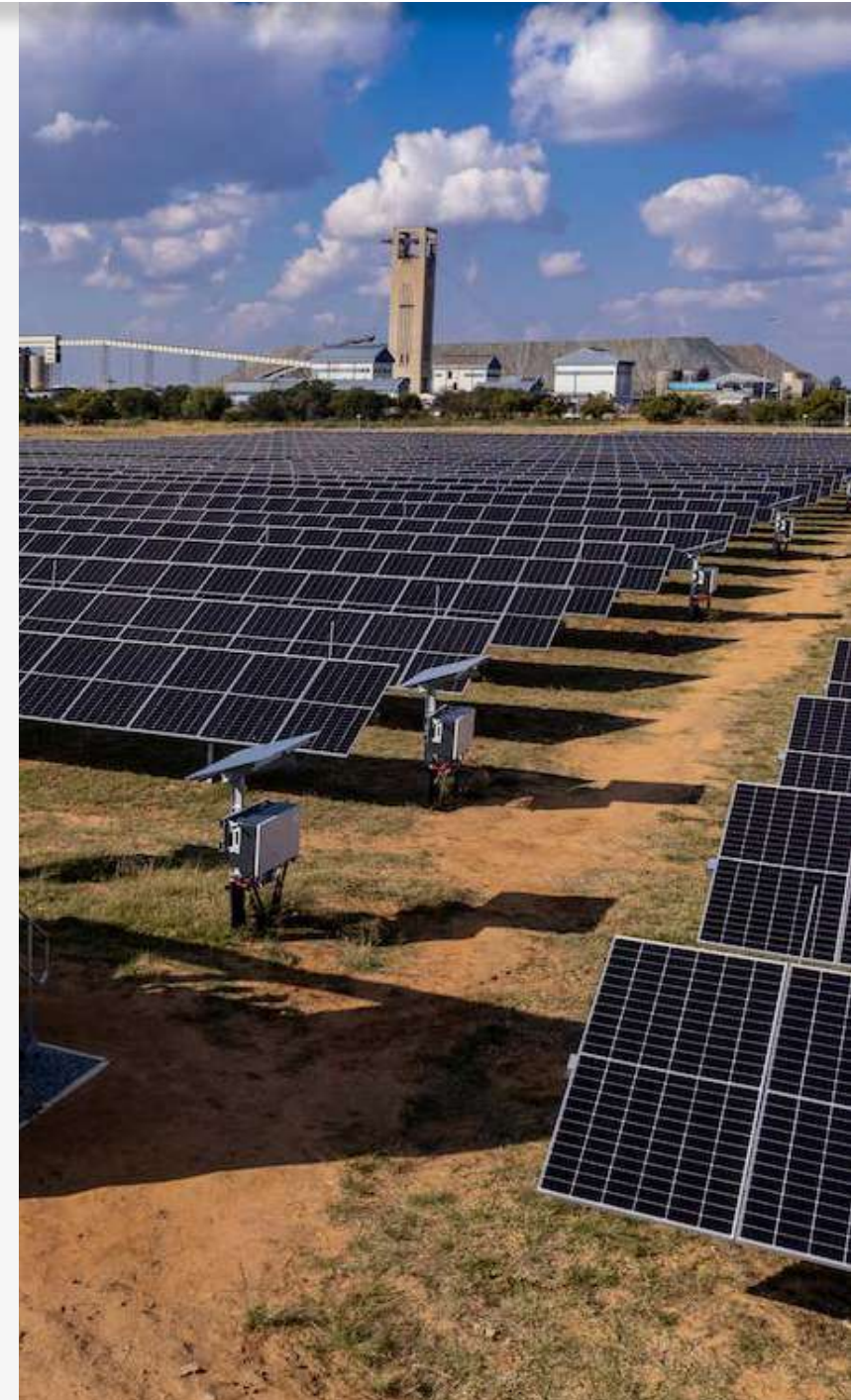
Tshepong solar plant
